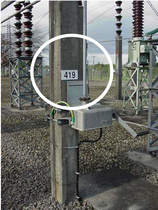
Figure C3: Label on pillar at a line earth switch operating position
