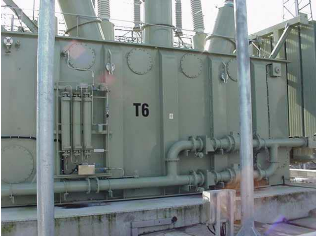
Figure C5: Transformer - label position
