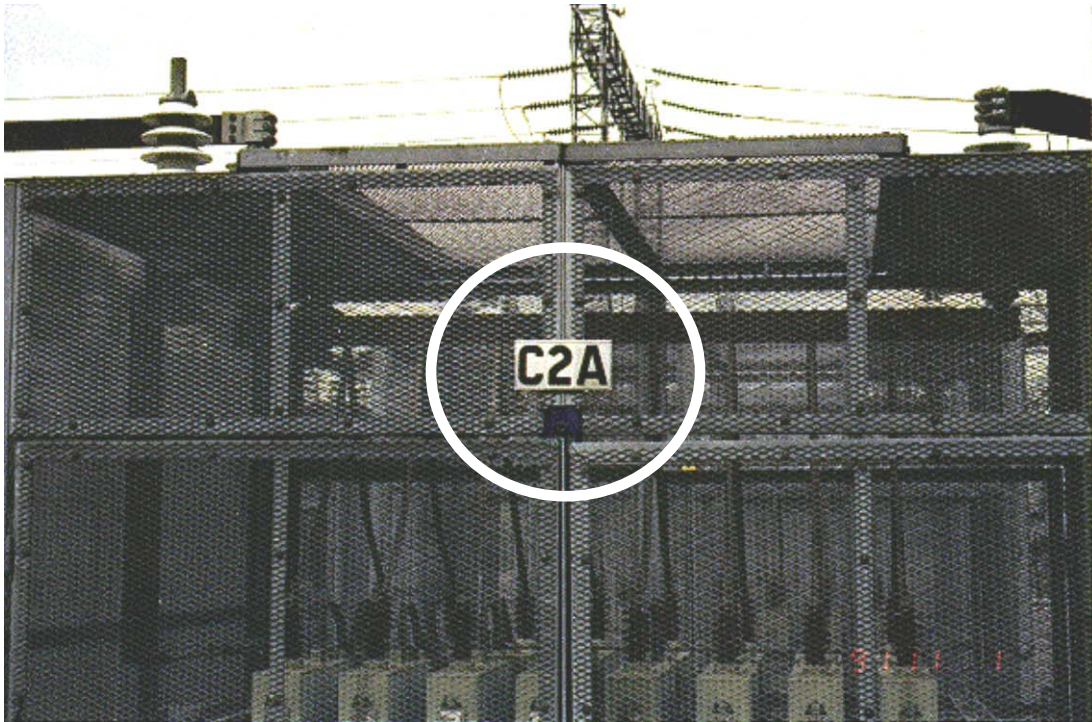
Figure C4: Labelling at the entrance of a capacitor bank enclosure
