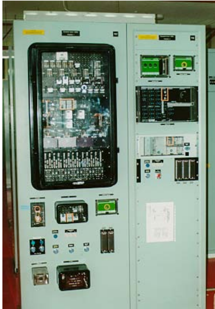
Figure 1: Typical Relay Cabinet with Protection Labeling
